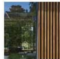
Timber fins in front of glazing to provide operable vents and solar shading
